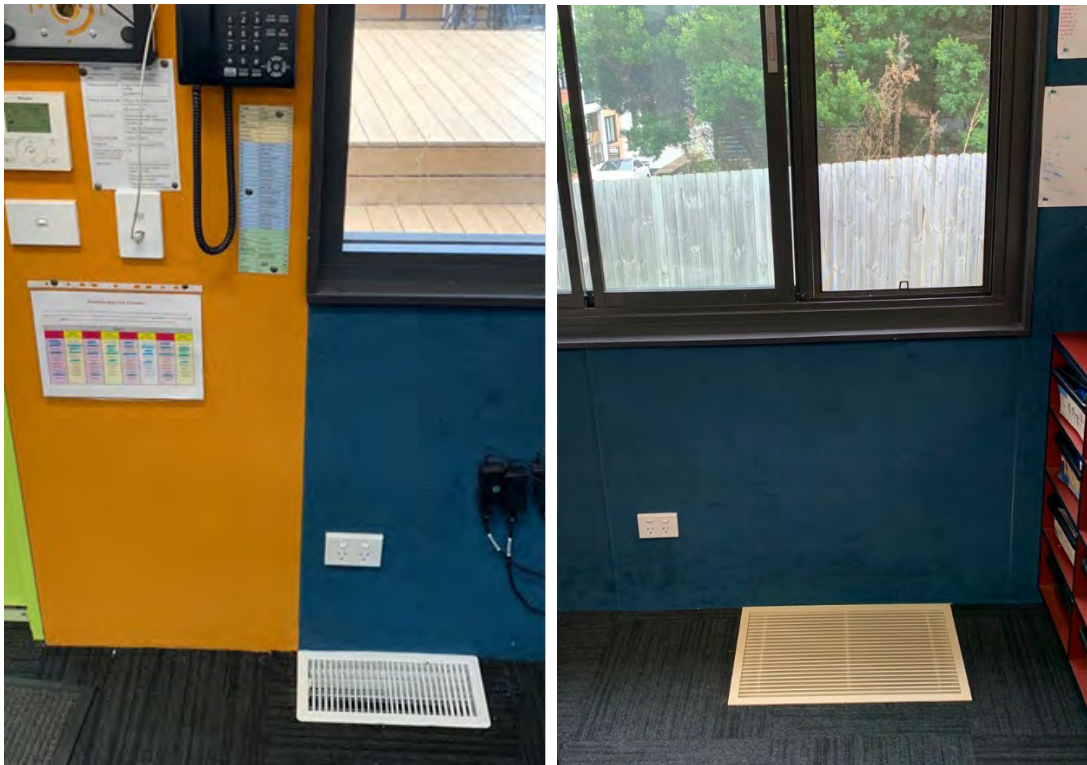
Figure 5-6. Installation photos for St Felix, showing the supply (left) and return (right) vents connected with the underfloor HRV unit.
