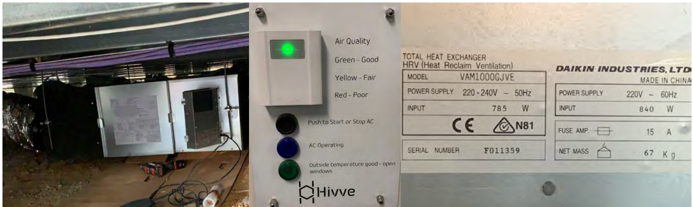
Figure 5-1. As installed images of the HRV unit at Majura in the ACT.
