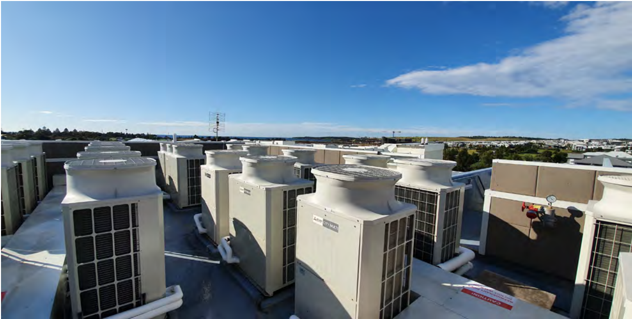
Figure 3-2 - Roof top Mitsubishi City Multi VRF HVAC units
