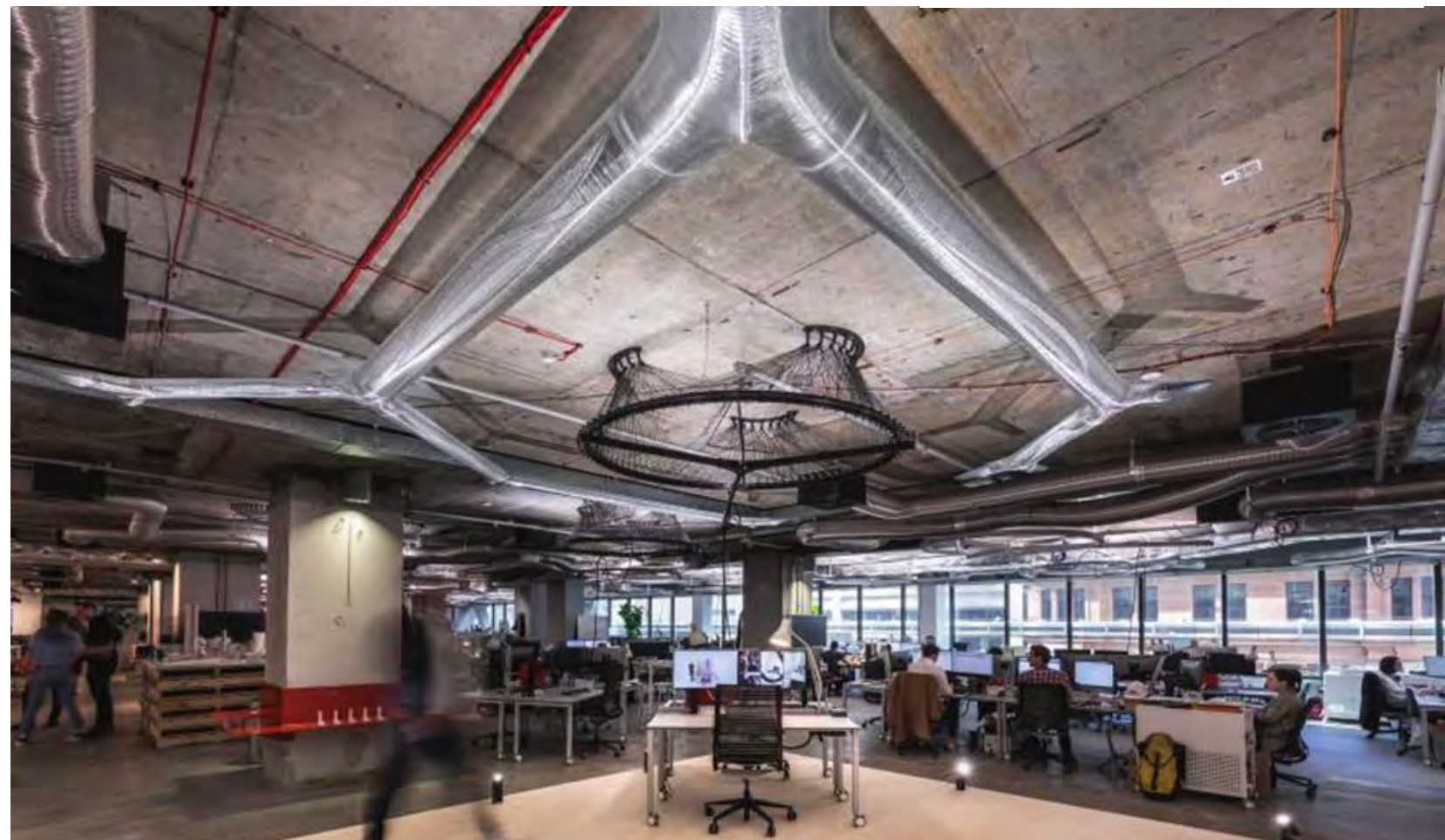
3D Printed Ductwork in BVN's Offices: https://www.hvacnews.com.au/news/is-this-the-hvac-system-of-the-future/
