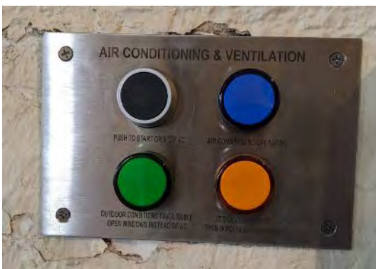
Figure 11: Financial modelling - CCP HVAC control panel
