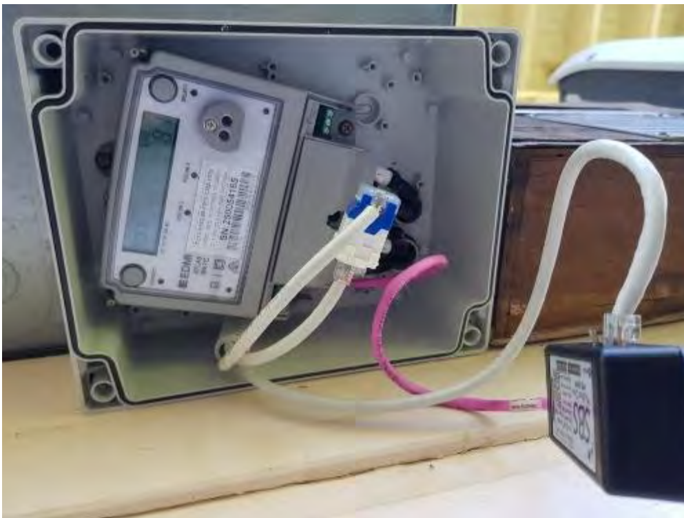
Figure 13: living lab - EDM1 utility meter and modbus RTU adaptor
