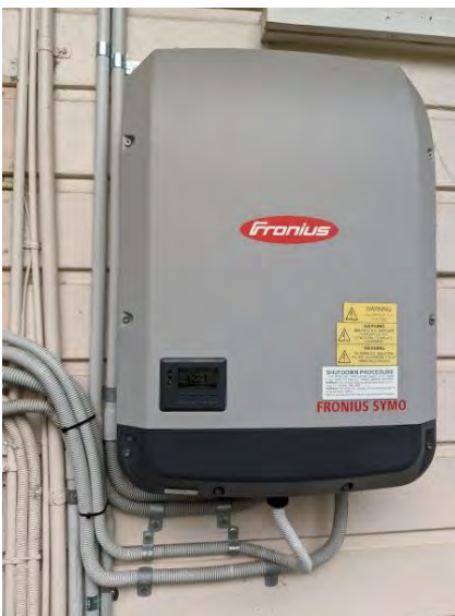
Figure 11: - Fronius solar PV inverter via modbus TCP
