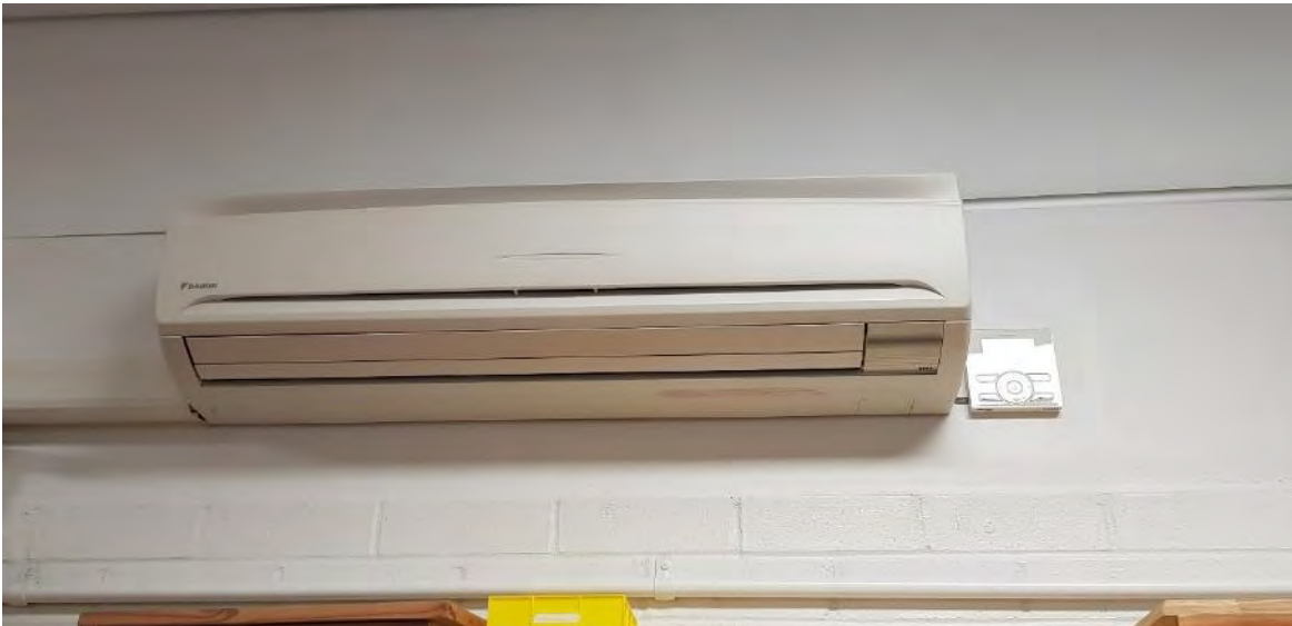
Figure 64: site report - Jamison HS typical Daikin FCU
