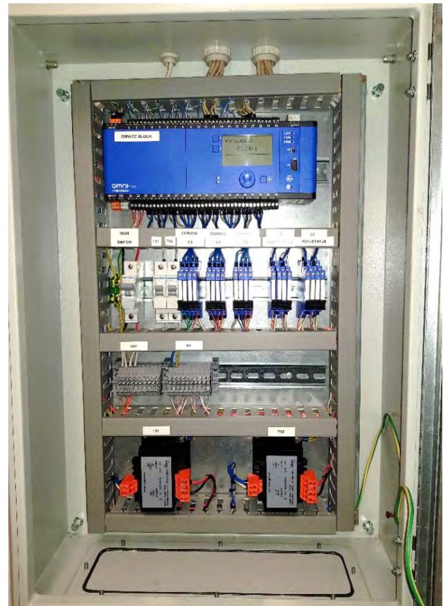
Drawing 5: site report - Nimbin CS typical CCP HVAC control panel
