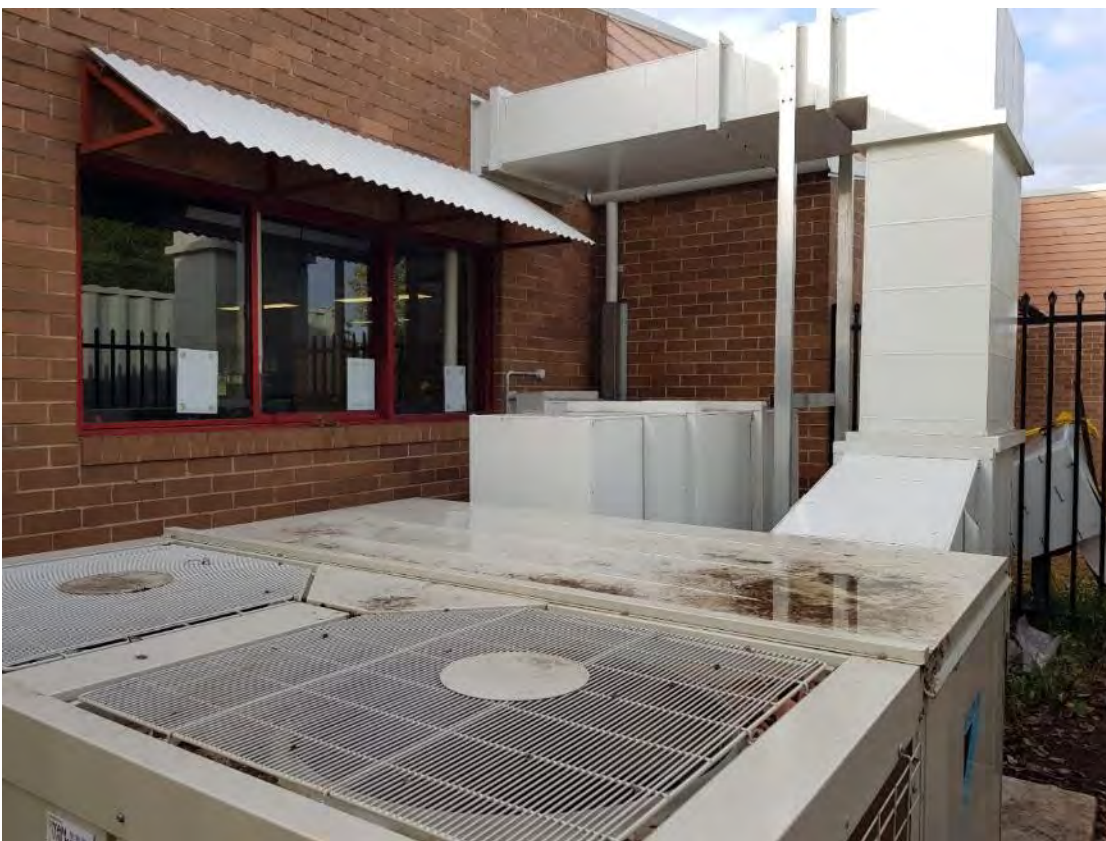
Figure 65: site report - Jamison HS typical Daikin condenser unit (with return air)
