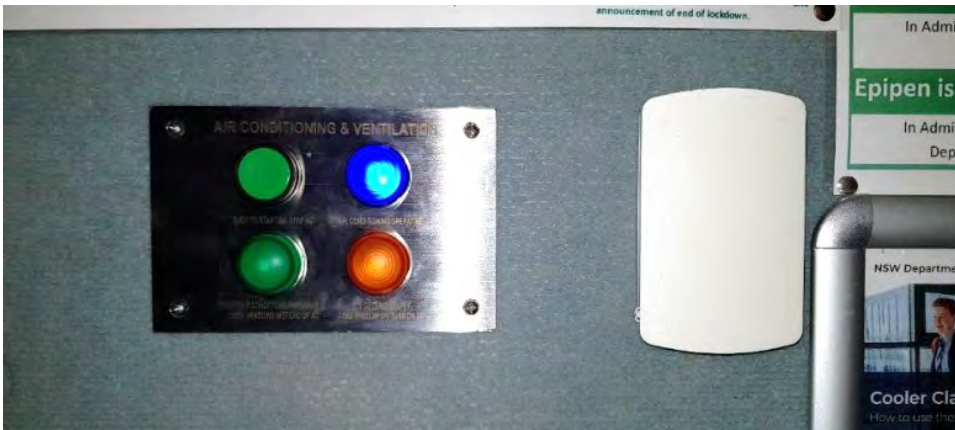
Figure 75: site visit - Nimbin CS typical CCP HVAC control panel, and temp/CO2 sensor
