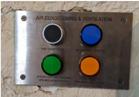
Figure 155: financial modelling - CCP HVAC control panel
