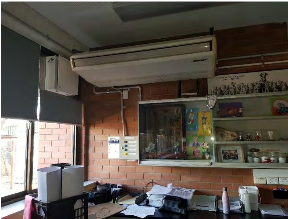
Figure 70: site report - Singleton HS typical HVAC system
