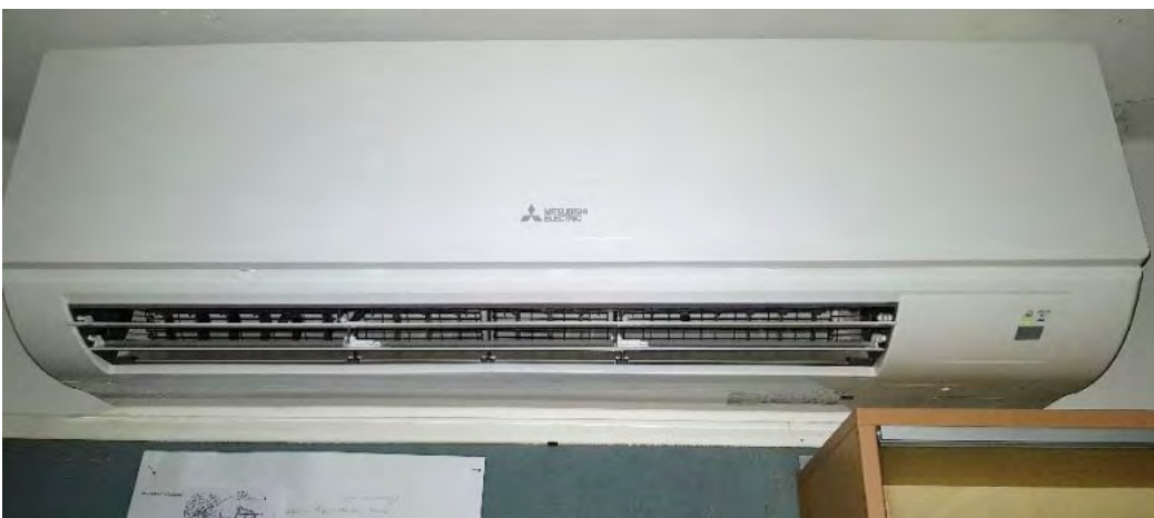
Figure 74: site report - Nimbin CS typical Mitsubishi 'city multi' FCU
