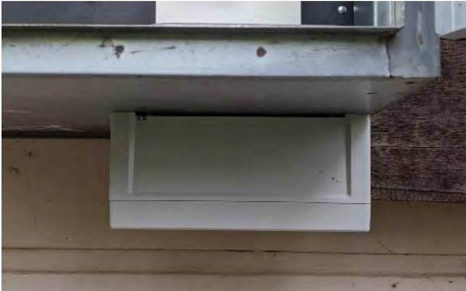
Figure 12: living lab - private EDM1 meter located below main meter panel
