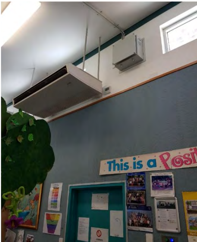
Drawing 4: site report - Nimbin CS library showing FCU, control panel and ventilation fan
