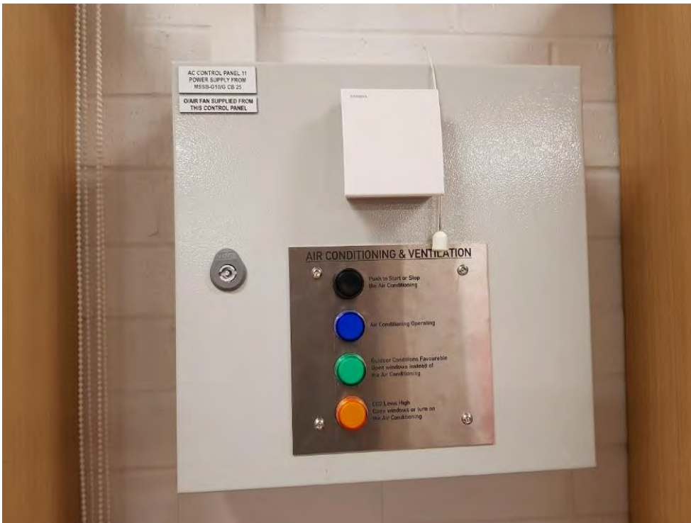
Figure 66: site report - Jamison HS typical CCP HVAC control panel
