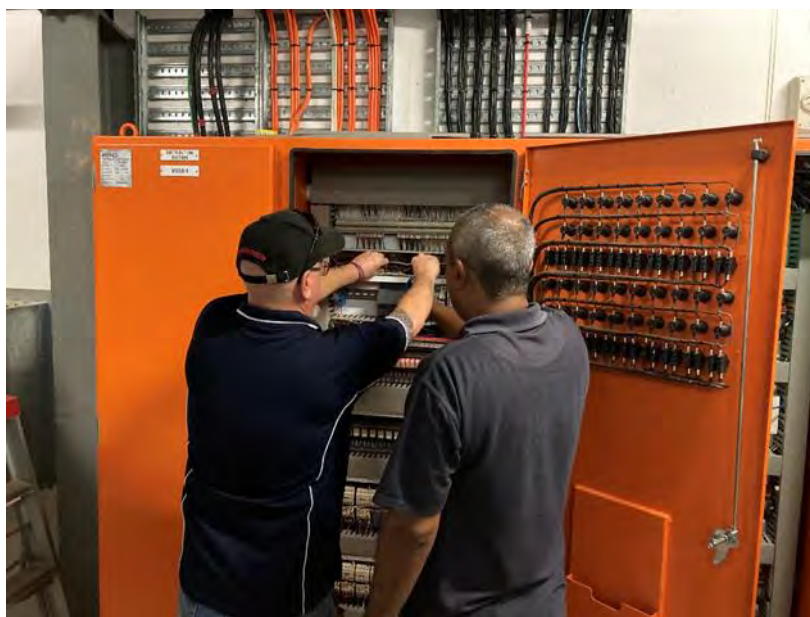
Figure 3: Installation of JACE gateway at Building Pink 9 (CDU)
