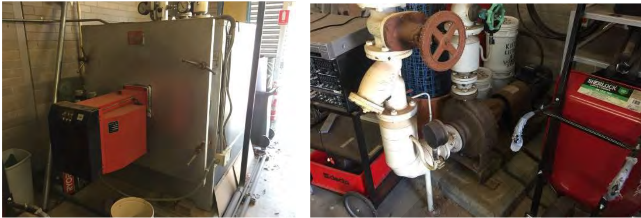
Figure 16: Central boiler and hydronic recirculation pump serving the Fadden Primary School site.
