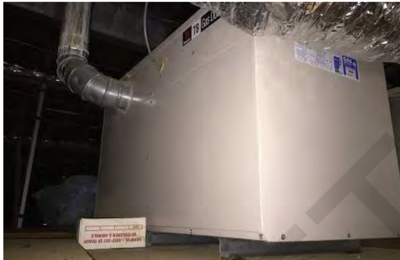
Figure 7: Amaroo preschool gas furnace for ducted heating of B12 only.
