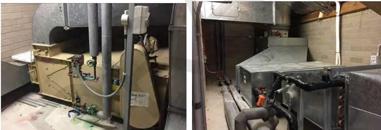
Figure 17: Air handling units: a) A typical original air-handling units serving the learning pods mounted above the entry foyer; b) A recently replaced air-handling unit.
