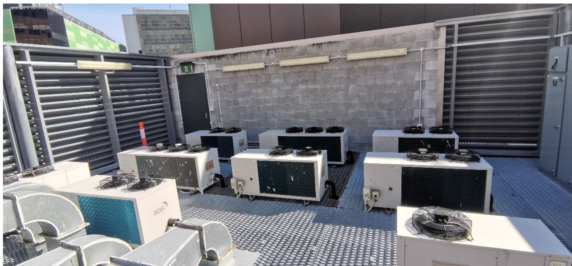
Figure 2 QCH Main Hospital Outdoor Plant Room
