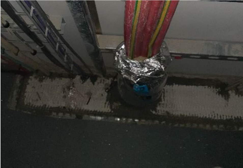
Figure 3-18 Sealed floor penetrations in electrical cupboards
