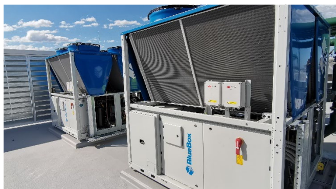
Figure 2-6 HVAC system chillers
