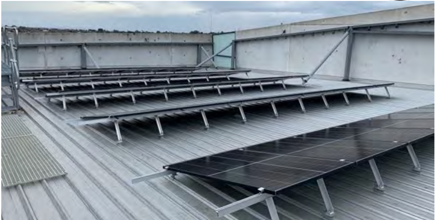
Figure 4: Installed PV system in the ATC roof top
