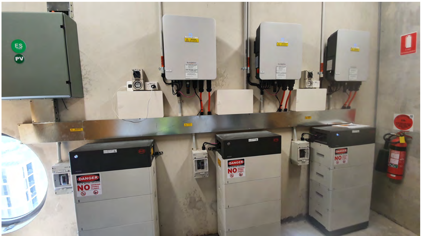
Figure 6: Inverter Room with 3 SH10RT inverters and Batteries
